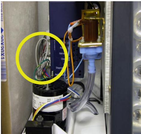
Unbundle gray wires for more slack, so photo-eyes can be pulled out.
