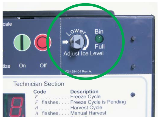
Ultrasonic control shown in its installed position, set at maximum fill.
