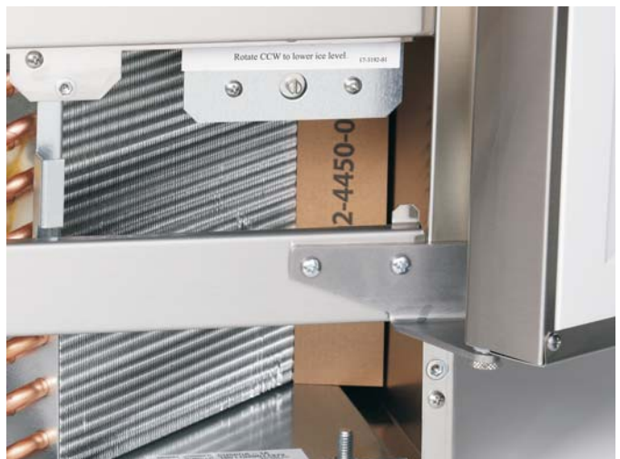
Condenser and Bin Thermostat
